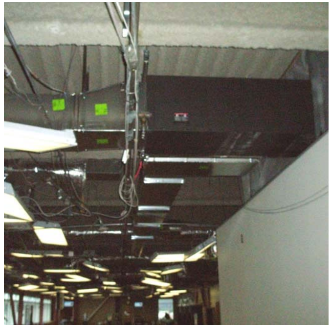
New Heat Pump in the Departure Lounge.
