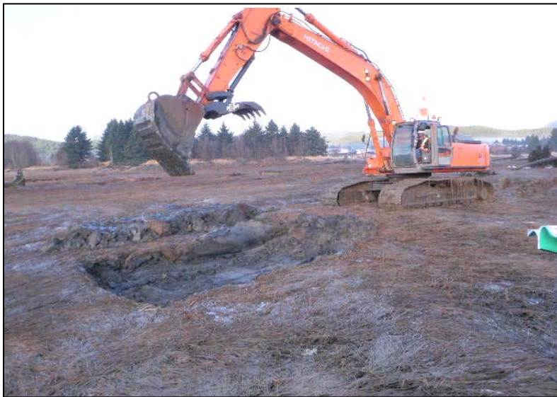
Placement of unsuitable material on West End Wetlands Fill area to determine how it reacts to tidal inundation.
