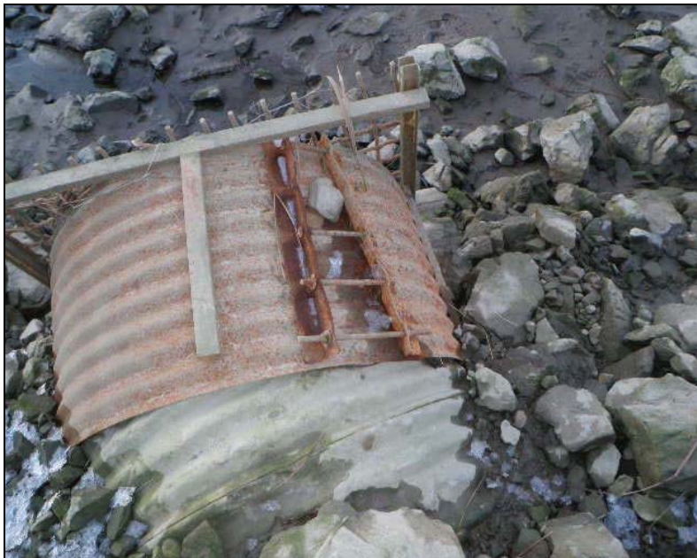
Float Plane Pond culvert that will be lengthened when we extend the Mendenhall River rip-rap armoring from the current project limit to the southwest corner of float plane pond.
