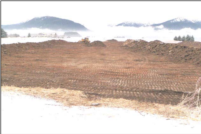
Stripping organic layer from NE Development Area. Good material exists just below the organic layer.
