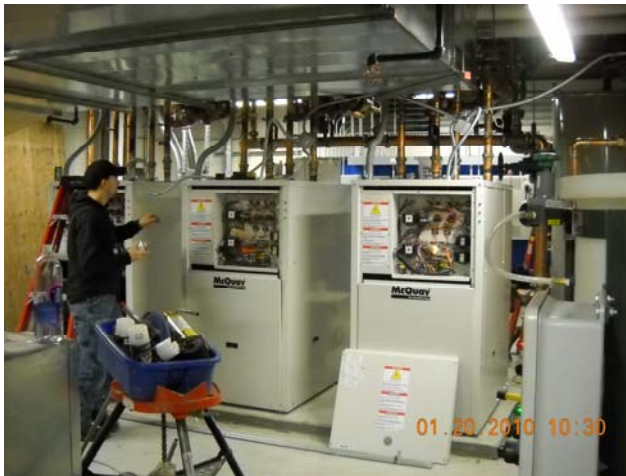
Heat pumps for geothermal system
