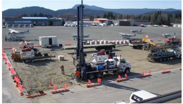
4.29.09: First day of drilling. Gregory Drilling constructed a total of 108 bore holes, each to a depth of 360 ft.
