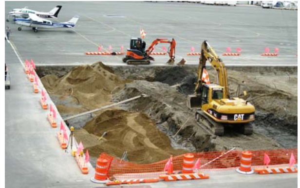
6.25.09: Trenching between rows of borings is complete; bedding material will be spread to rest the horizontal pipes upon. Note the existing conduits that will remain in place.
