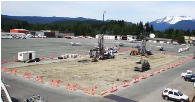
6.4.09: Drilling is nearly complete. U-bend assemblies of 3/4" HDPE pipe were set in each hole, and backfilled with pea rock.
