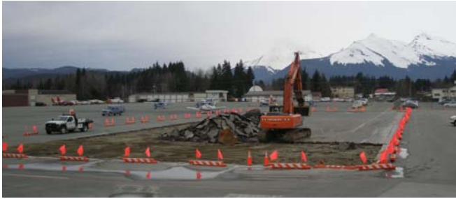
4.16.09: Asphalt removal underway by Admiralty. Cones mark the perimeter of the loop field, a 100 ft x 300 ft. area.
