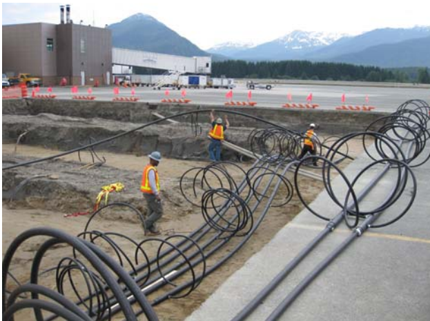
7.02.09: Manifolds are moved onto the site by Harri's Plumbing & Heating crew. Each pipe assembly was pre-assembled with fused joints off-site.
