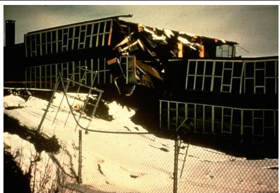
Earthquake damage to buildings in Anchorage, Alaska after the 1964 earthquake.
