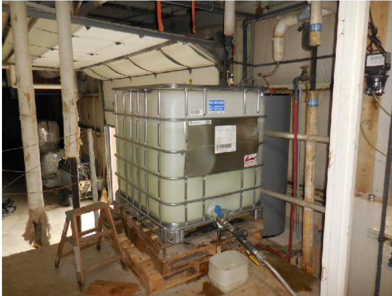
Figure 15. Polymer Addition Area
