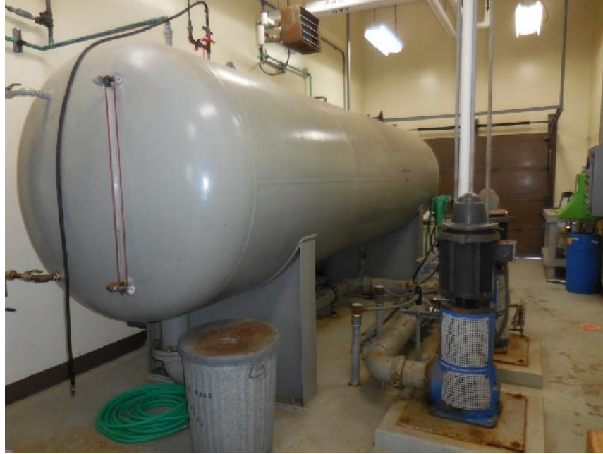
Figure 11. NPW Tank and Pump System
