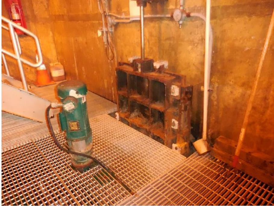
Figure 3. Influent Gate Valve
