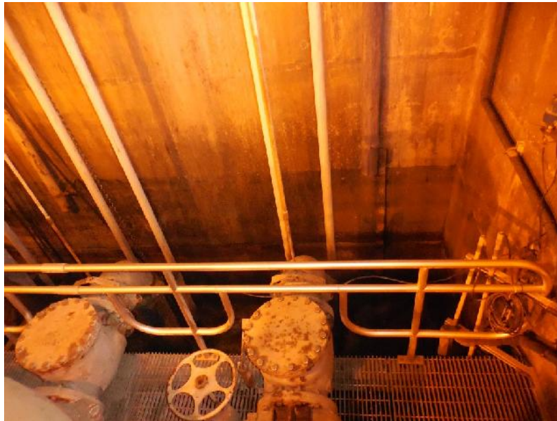
Figure 5. IPS Wet Well
