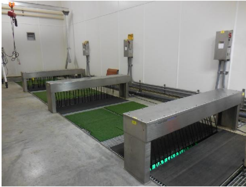
Figure 10. UV Disinfection System
