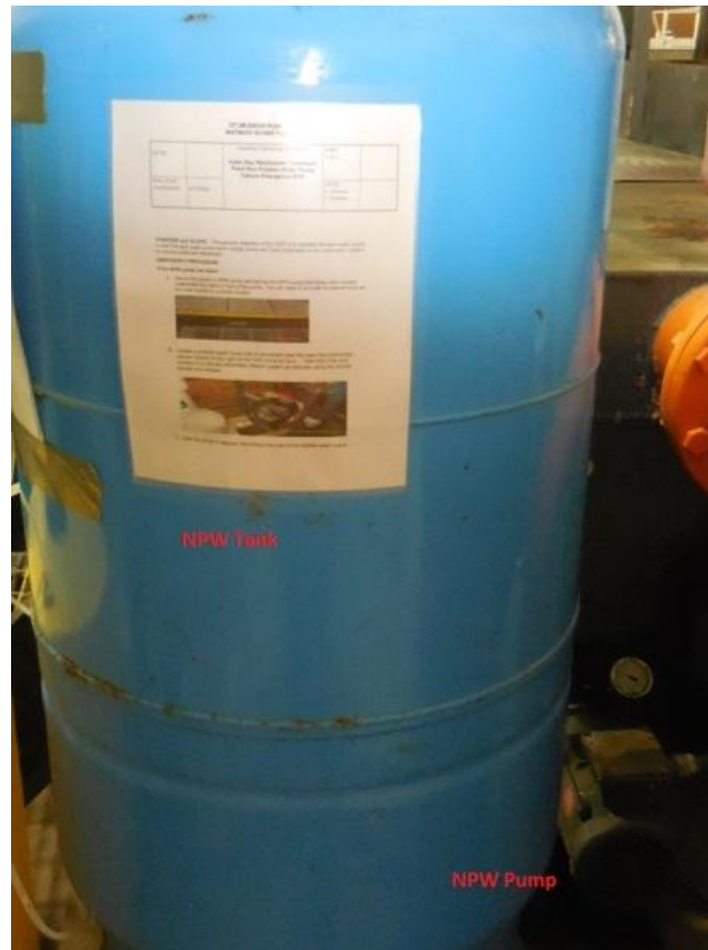
Figure 10. ABTP NPW pneumatic expansion tank and pump
