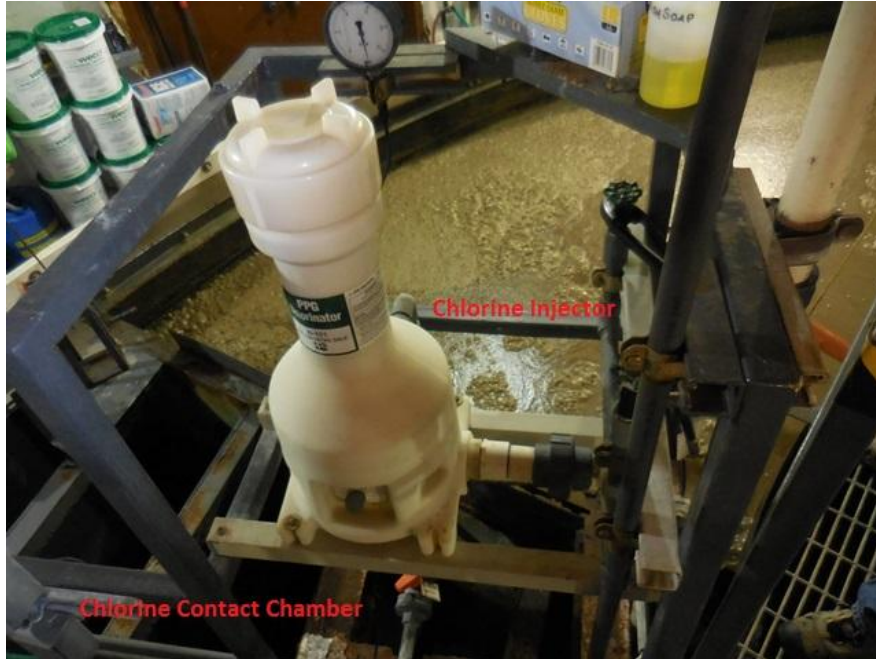
Figure 8. ABTP Chlorine Contact Chamber
