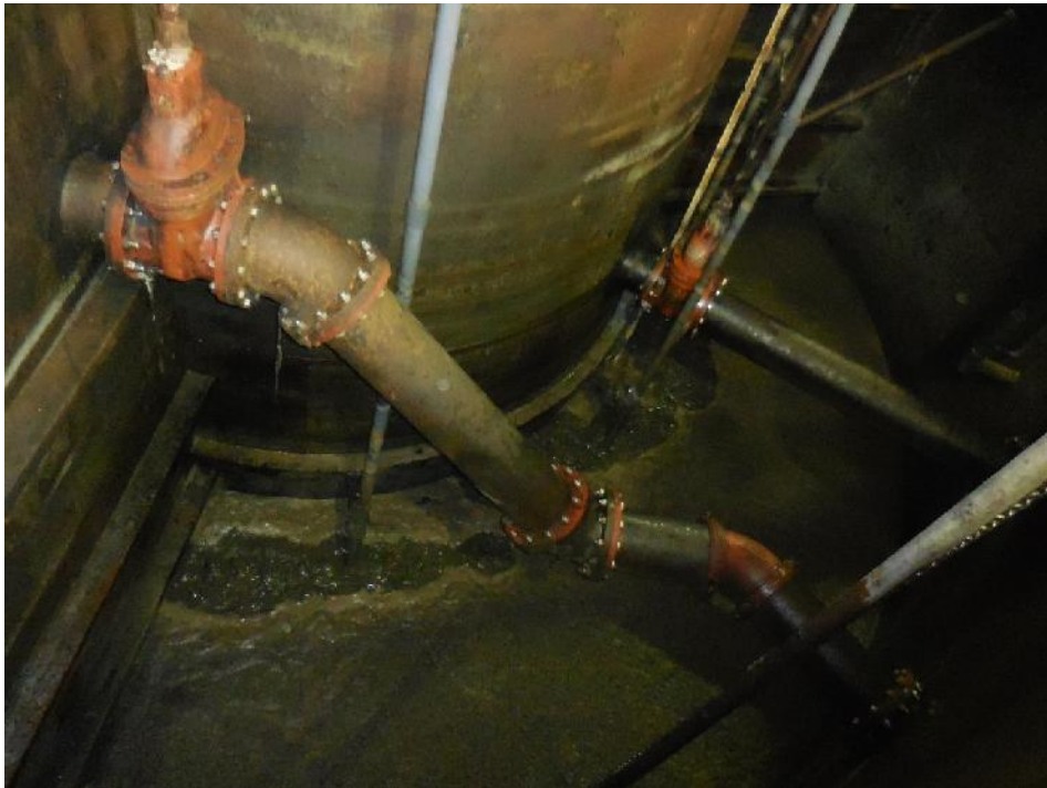
Figure 11. ABTP Solids Holding Tank
