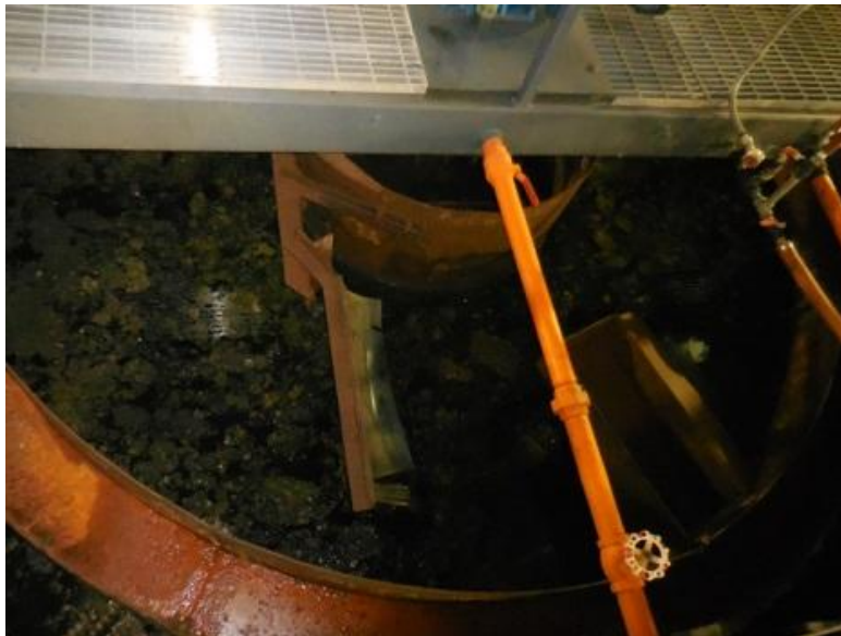
Figure 6. ABTP Secondary "Polishing" Clarifier
