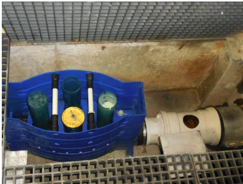
Figure 9. ABTP Sodium Sulfite Feeder
