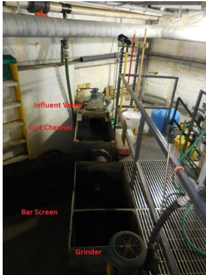
Figure 3. ABTP Preliminary Treatment Headworks
