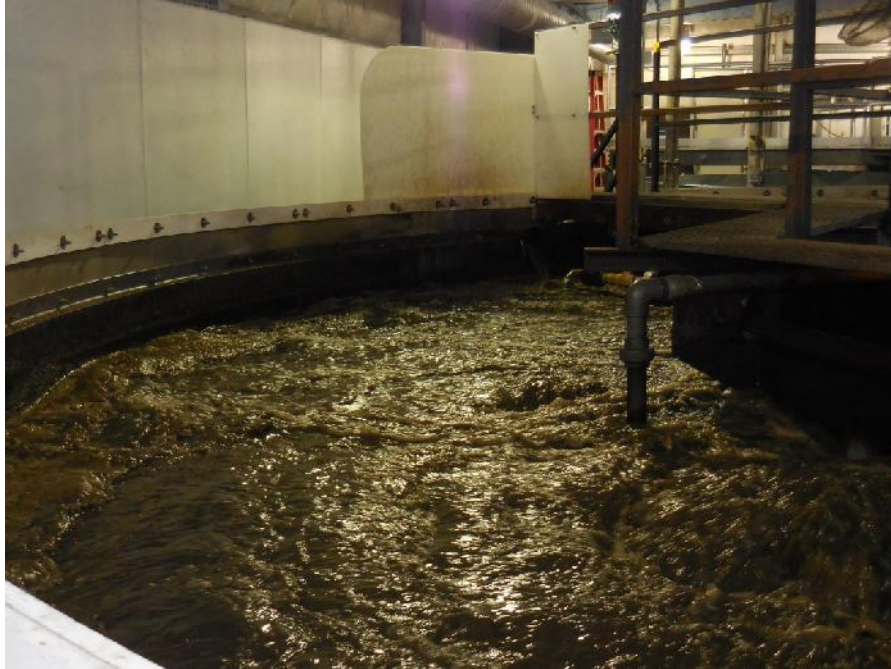
Figure 7. ABTP Reaeration Basin
