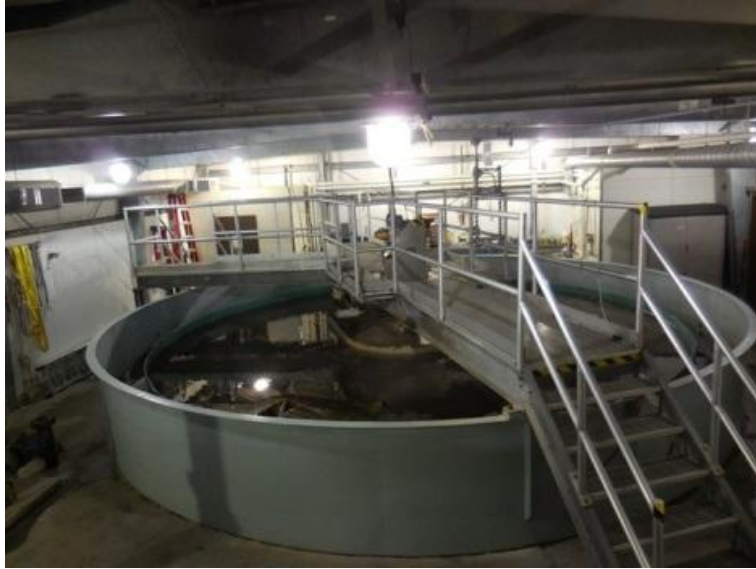
Figure 5. ABTP Secondary Clarifier
