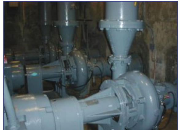
Lift stations move sewage from areas of lower elevation to higher elevation. The replacement of the Valley Court sewer main and the Gruening Park lift station are estimated to cost $1.5 million.
