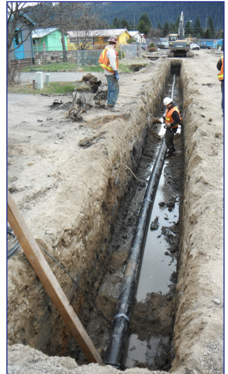
Crews install a new 8-inch water main in Eagles Edge Subdivision this spring.
