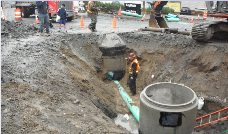
Crews install the sanitary sewer system along Main Street last summer. The large concrete structures will house the man holes that provide maintenance crews access for maintenance and repairs.
