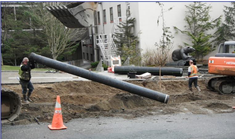
Water and sewer lines are usually located under roadways, so repairs and replacement are often done at the same time as road construction so that the road does not have to be torn up and repaved later. Here crews build a new water main under Juneau's Main Street last summer.
