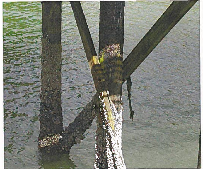
AURORA 010.jpg BROKEN X-BRACING ON "A" GANGWAY APPROACH DOCK
