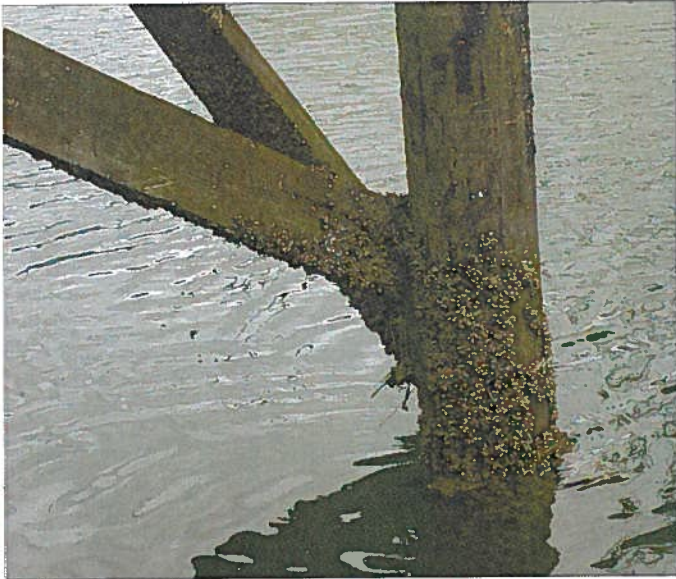
AURORA 019.jpg BROKEN X-BRACING AT "C" GANGWAY APPROACH DOCK
