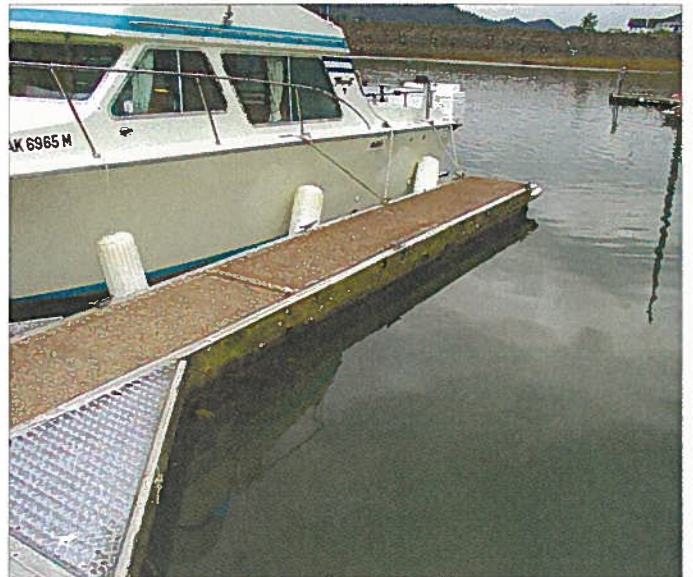
AURORA 096.jpg DETERIORATED TIMBERS ON FINGER ON "K" FLOAT
