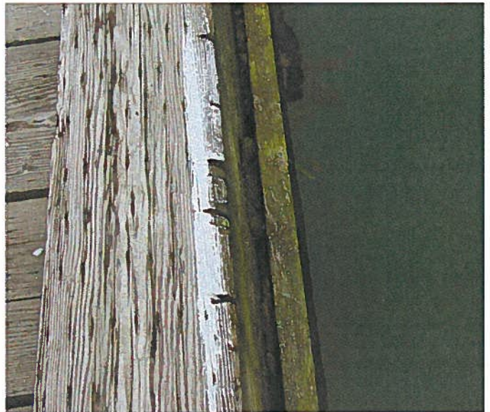
AURORA 046.jpg ROTTEN, DETACHED RUBSTRIP ALONG HEADWALK FLOAT. NEAR "D" FLOAT
