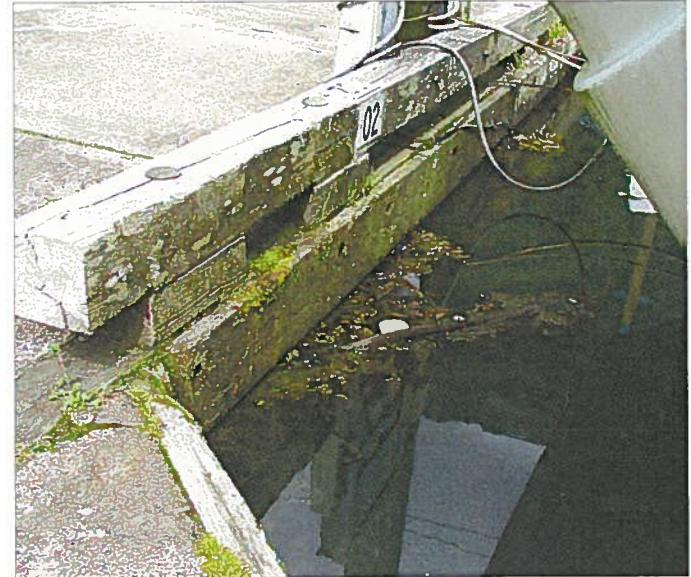
AURORA 084.jpg LOW FREEBOARD ON "G" FLOAT
