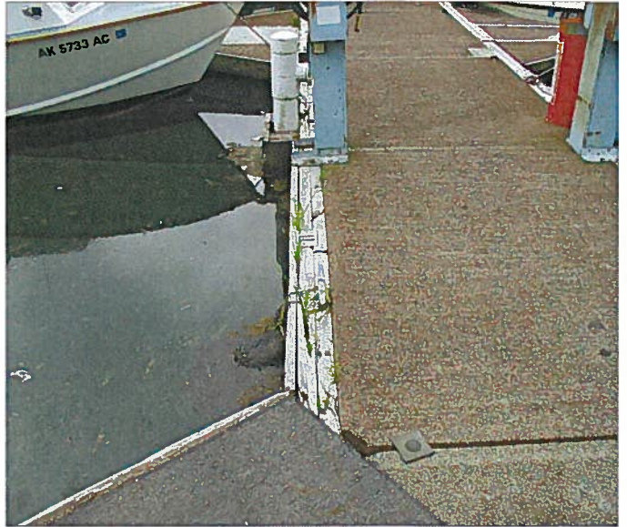
AURORA 106.jpg VEGETATION/DETERIORATED FLOAT TIMBERS ON "N" FLOAT
