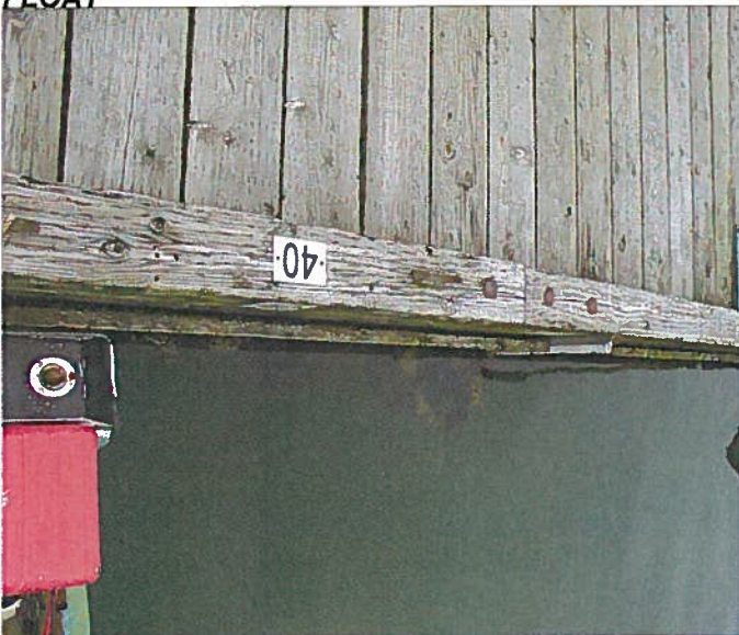
AURORA 045.jpg ROTTEN, DETACHED RUBSTRIP ALONG HEADWALK FLOAT. NEAR "D" FLOAT
