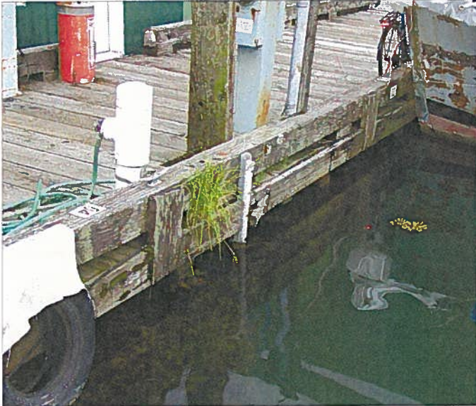
AURORA 079.jpg ROT, DETERIORATED RUBSTRIP AND VEGETATION ON "E" FLOAT
