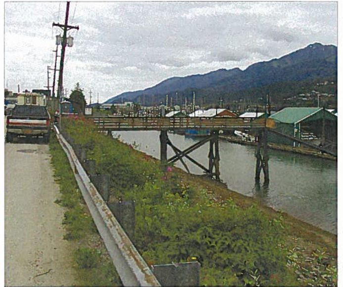
AURORA 034.jpg DAMAGED BRACING AT "H" APPROACH DOCK
