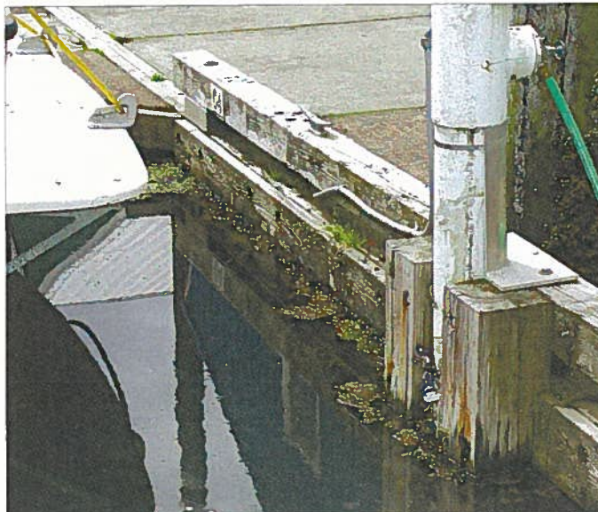
AURORA 083.jpg LOW FREEBOARD ON "G" FLOAT
