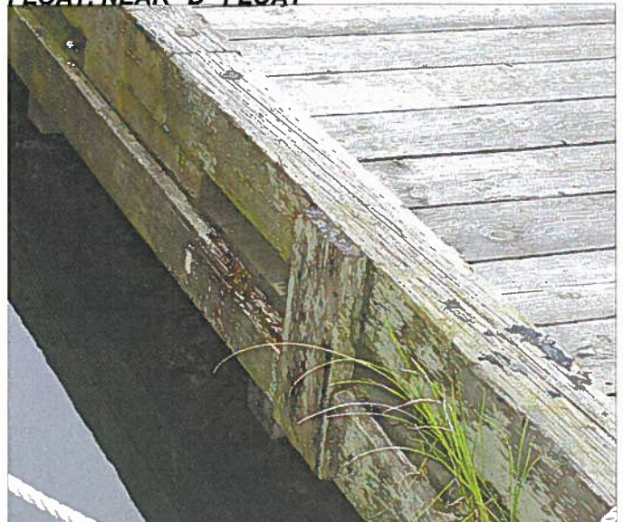
AURORA 048.jpg ROTTEN RUBSTRIP ALONG HEADWALK NEAR "A" FLOAT
