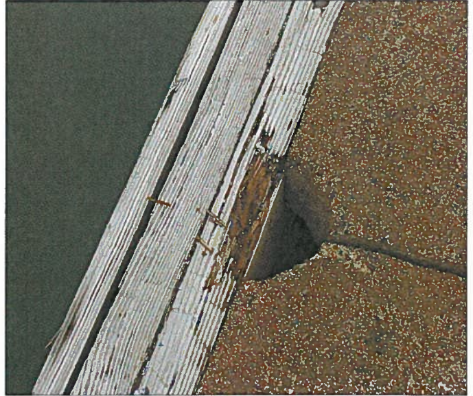
AURORA 050.jpg ROTTEN TIMBER WALERS ON HEADWALK FLOAT BETWEEN "H" AND "J" FLOAT
