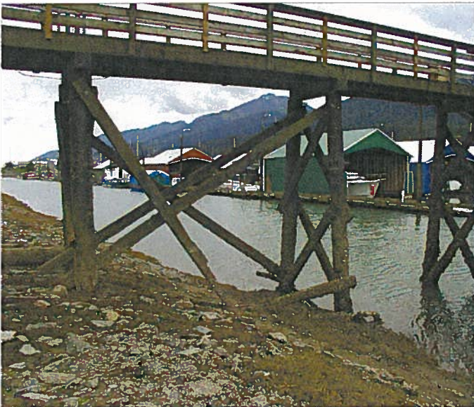
AURORA 033.jpg DAMAGED BRACING AT "H" APPROACH DOCK
