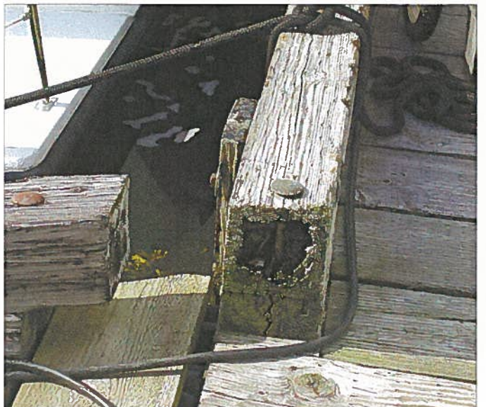
AURORA 066.jpg TYPICAL ROTTEN HEADWALK BULLRAIL
