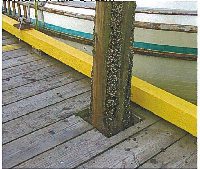
AURORA 052.jpg TYPICAL ABRADED HEADWALK PILE
