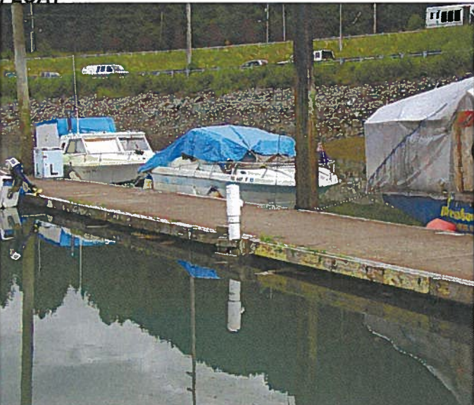
AURORA 041.jpg ROTTED TIMBER WALERS ON HEADWALK FLOAT BETWEEN "K" AND "L" FLOAT
