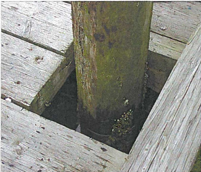
AURORA 073.jpg "C" FLOAT ABRASED PILE AND WORN RUB STRIPS
