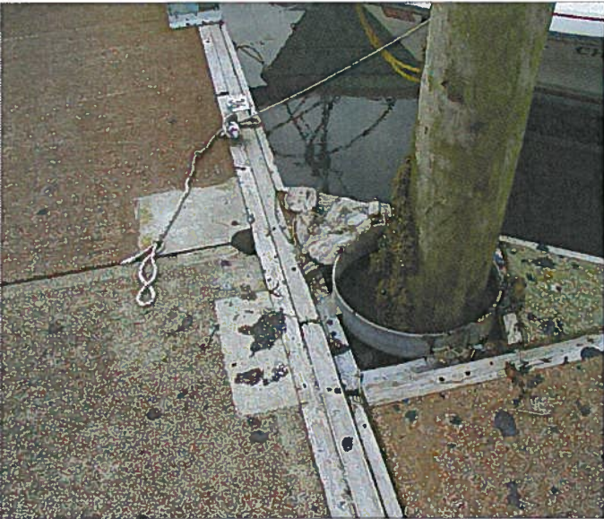
AURORA 105.jpg BROKEN WALER ON "N" FLOAT
