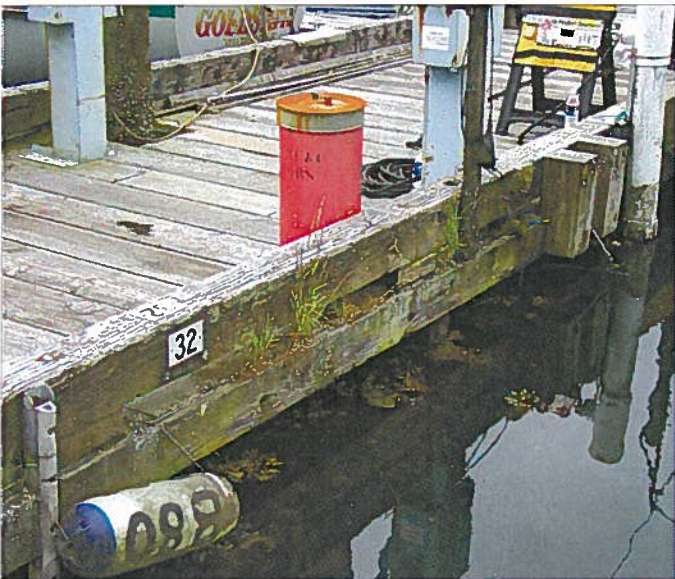
AURORA 075.jpg ROT AND VEGETATION ON "D" FLOAT
