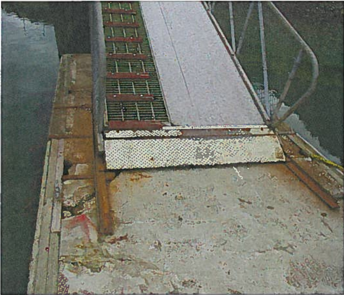
AURORA 057.jpg "N" GANGWAY/FLOAT TRANSITION, SKIDS, DETERIORATED LANDING FLOAT
