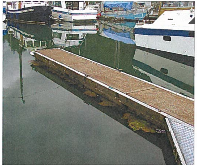
AURORA 098.jpg DETERIORATED TIMBERS ON FINGER ON "K" FLOAT
