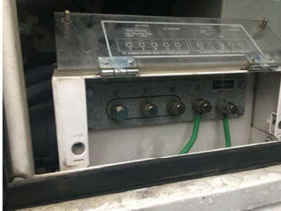
Figure 3: Terminal Block with Compression Connectors
