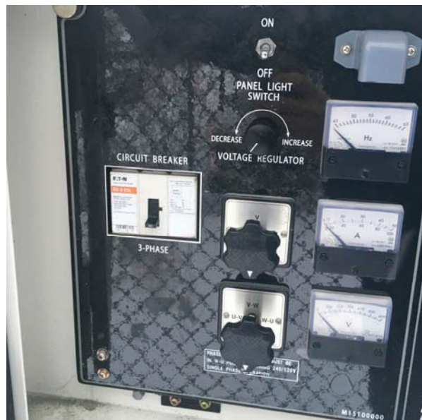
Figure 4: 60 Amp Circuit Breaker
