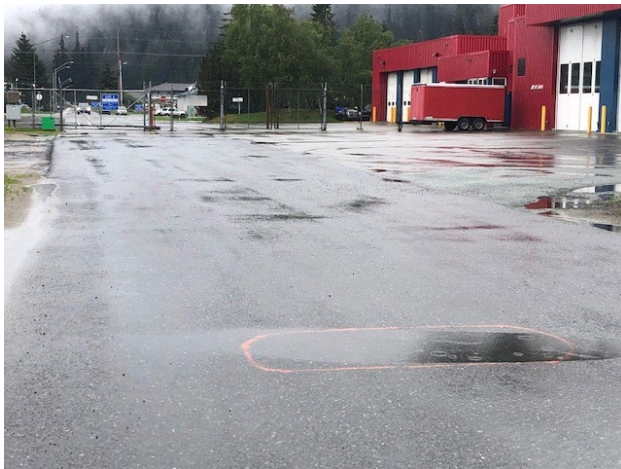
Photo 01: Depression in asphalt above the culvert.
