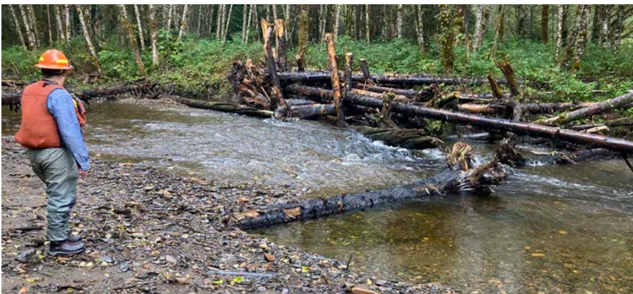
An example of a multi-tree structure assembled in a stream to improve salmon habitat in Margaret Creek on Revillagigedo Island near Ketchikan.
