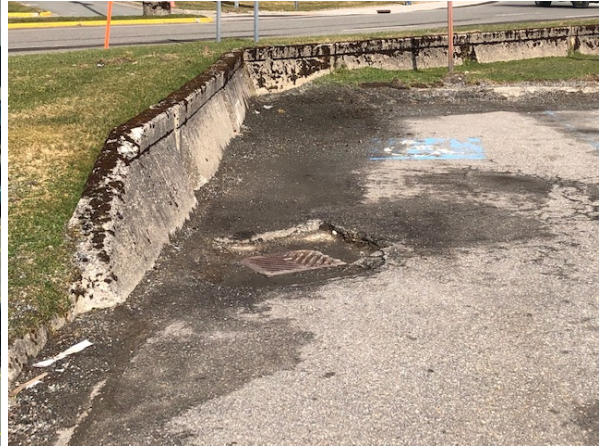
Long term parking lot failing vault
