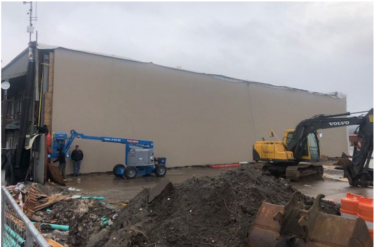
Photo 01: Southeast Earthmovers installing the last of the insulated metal panel siding over the new columns, beams and horizontal girts at the northwest corner of the Loken Hangar.
