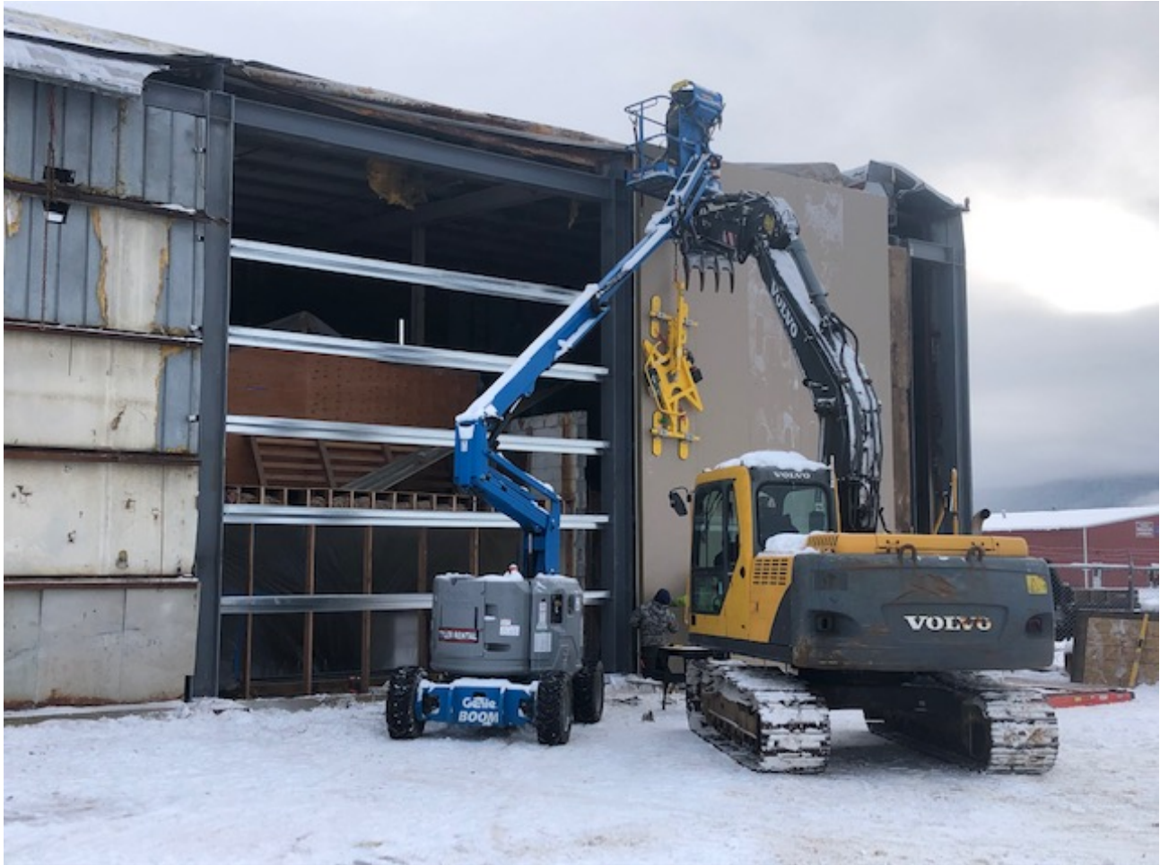
Photo 01: Southeast Earthmovers installing insulated metal panel siding over the new columns, beams and horizontal girts at the southwest corner of the Loken Hangar.
