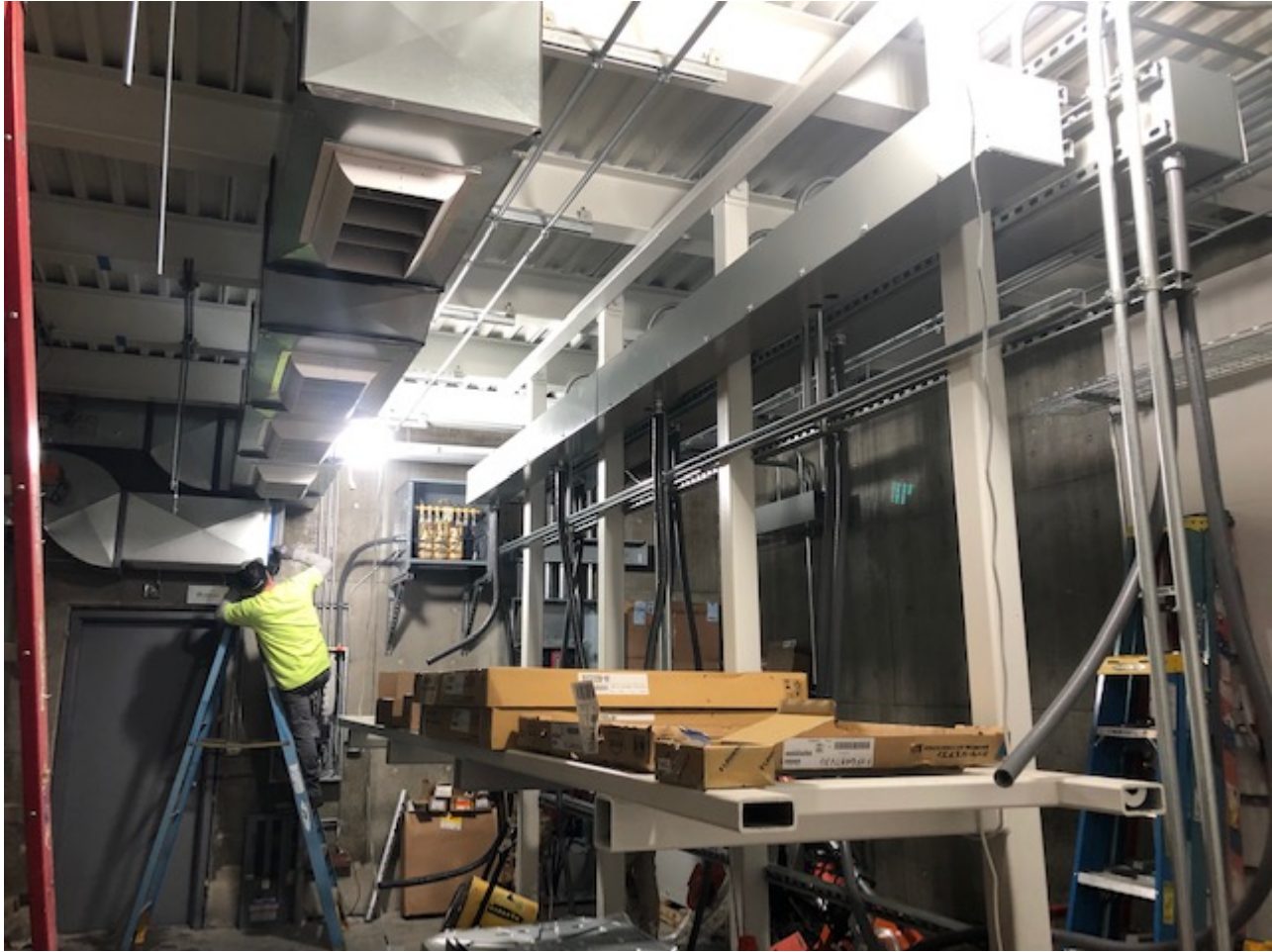
Photo 02: Return air ductwork being installed in the northwest corner of the new ALRV. The new regulator support rack is shown in the center of the photo.
