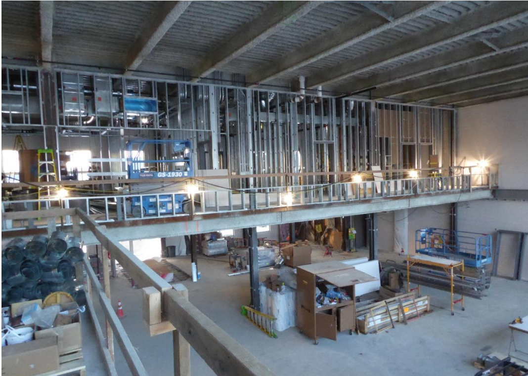
View toward airport admin suite & regional air carrier ticketing from stair tower balcony.
