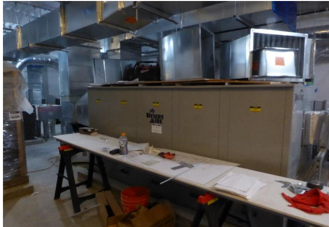
Air handler in penthouse.
