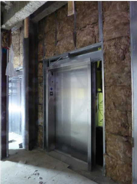
1 st floor elevator entrances.
