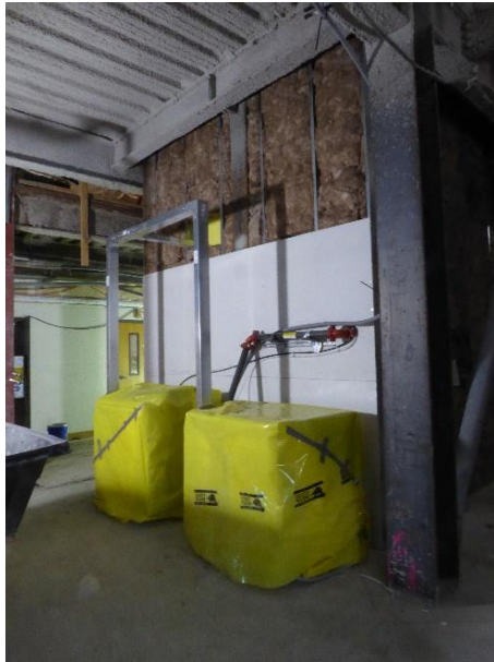
Elevator machinery on 1 st floor. (Protected with plastic wrap.)
