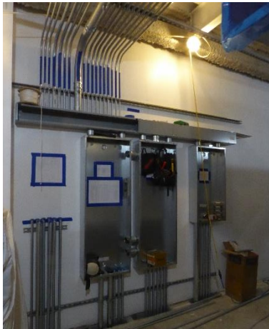
Penthouse electrical panels.
