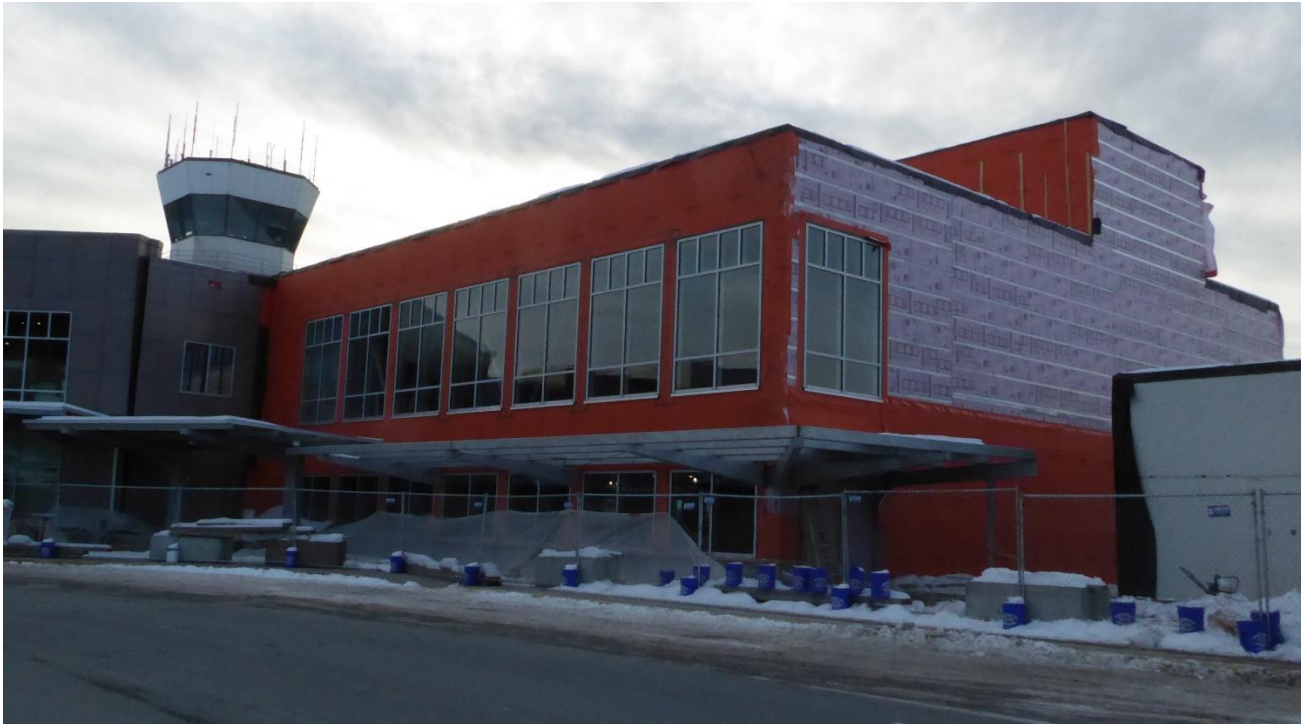
Terminal reconstructed building viewed from Shell Simmons Drive. (Air & water barrier installed over Z-girts with rigid insulation.)
