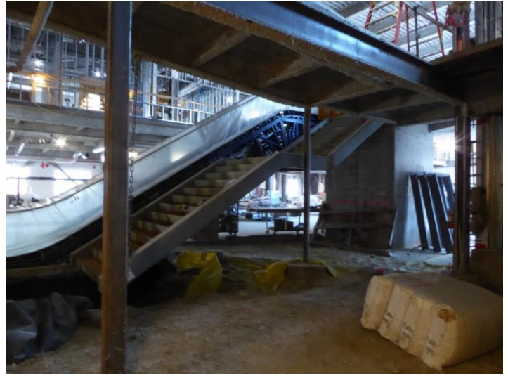
Escalator installed adjacent main stairway.
