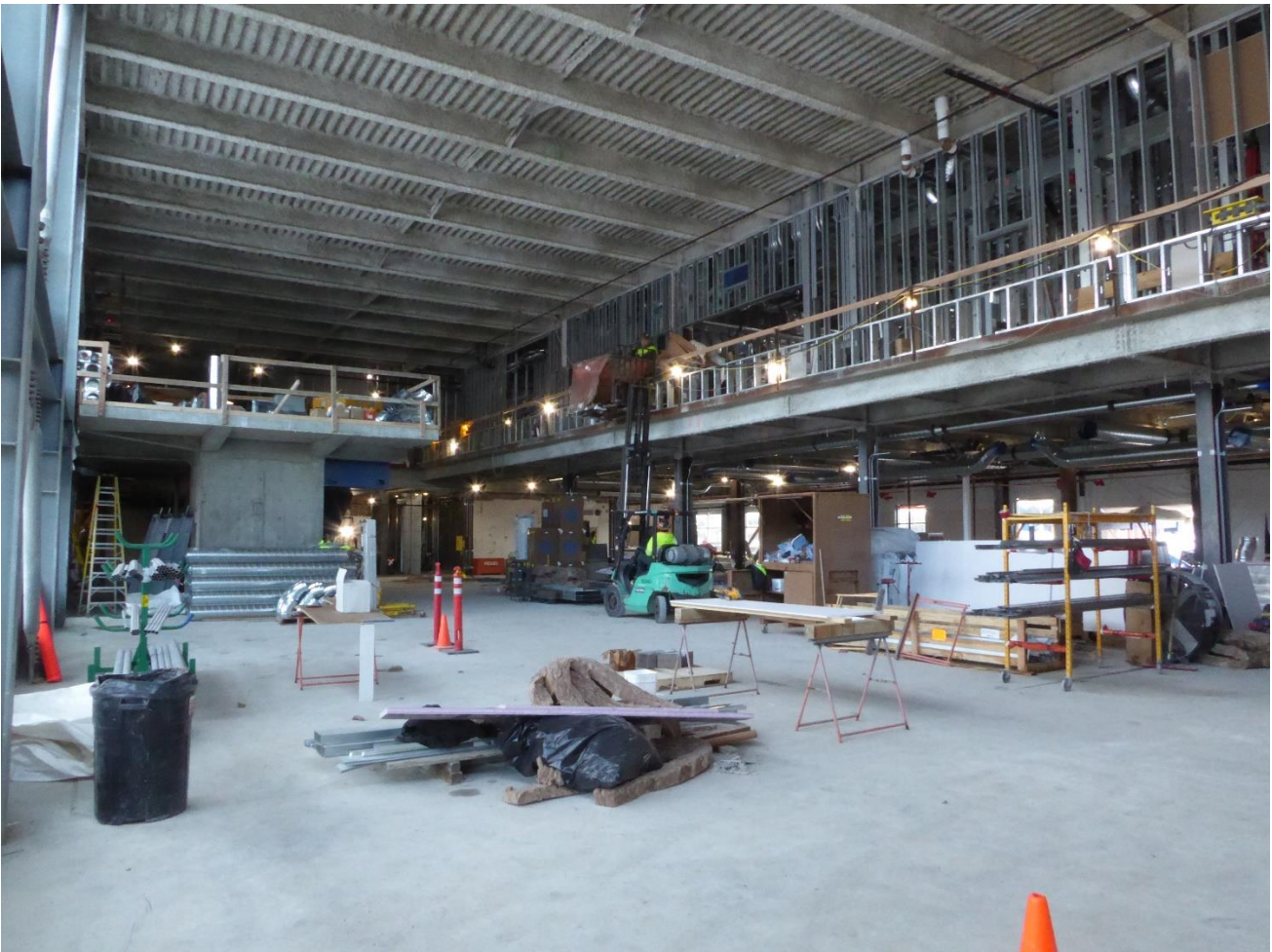
View from north vestibule area looking into regional air carrier seating space. (Stair tower to left — 2 nd floor balcony to right.)
