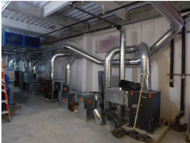
Heat pumps along west wall in penthouse.
