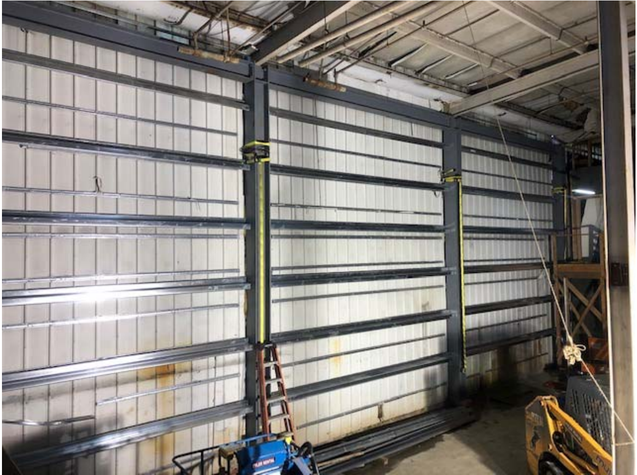
Photo 04: New columns, beams and horizontal girts in place. The old sand shed siding is visible behind the new work.
