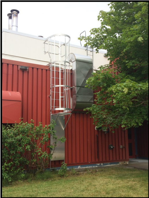
E. Façade- Cage Ladder & AHU-1 snorkel. Remove and Reinstall + all other accessories.
