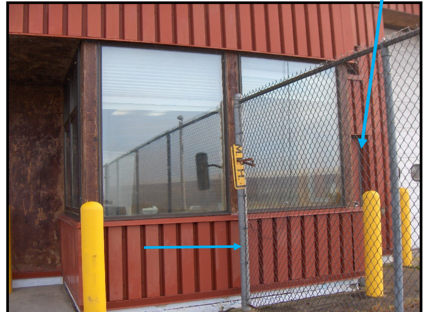
North— Dispatch office: SIDA fencing to be rolled up, secure w/Temp fencing. Note man-door on Right (arrowed) to be replaced is on SIDA side.
