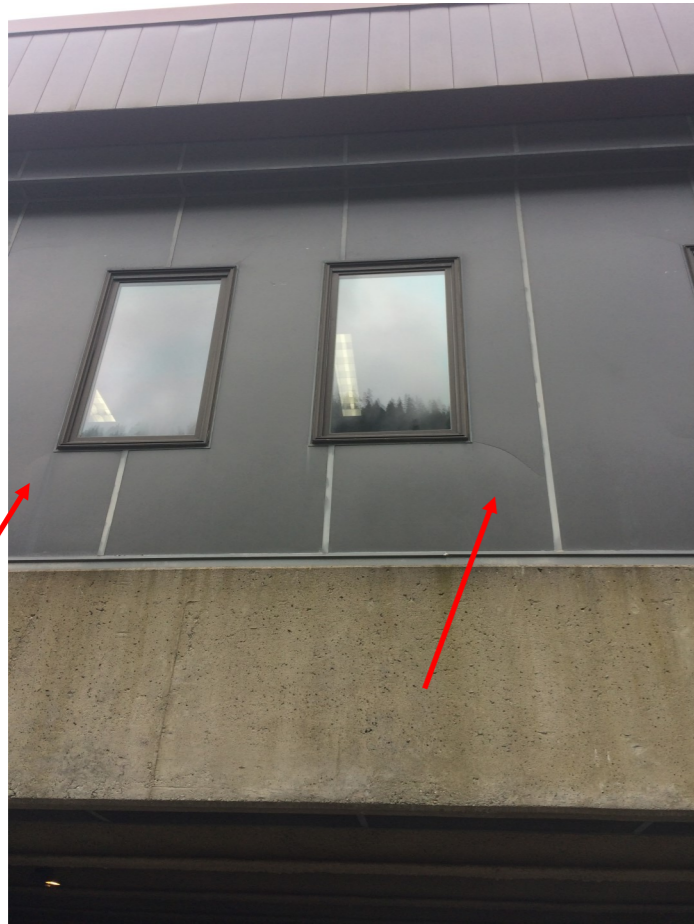
TYP. SIDING CRACKS AT WINDOW CORNERS
