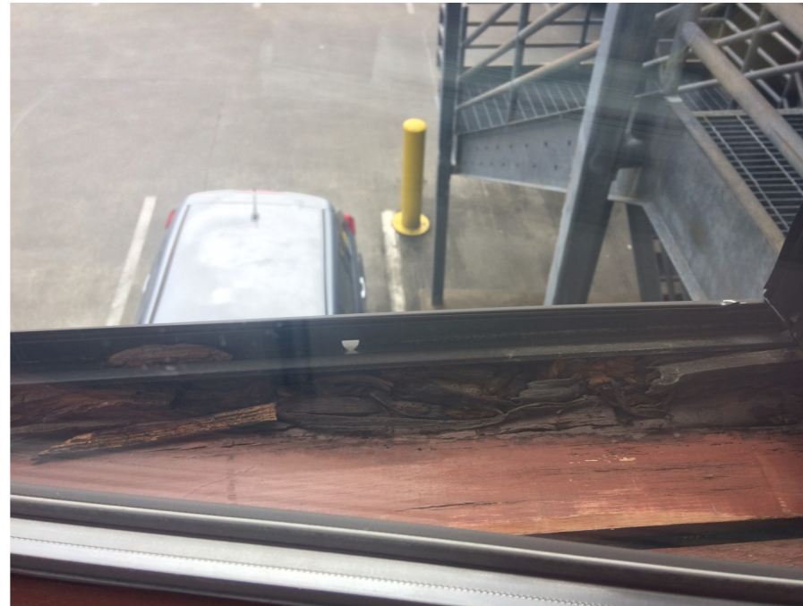
INTERIOR WOOD TRIM ROT—WINDOW SILL SOUTH FAÇADE—LEFT WINDOW CIRCLED BELOW
