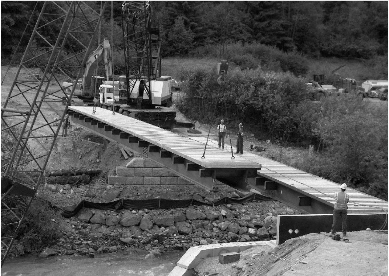
Lemon Creek Bridge - Photo By Bob Millard
