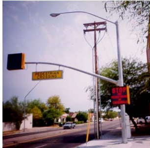
Figure 15 Crosswalk Overhead Illumination
