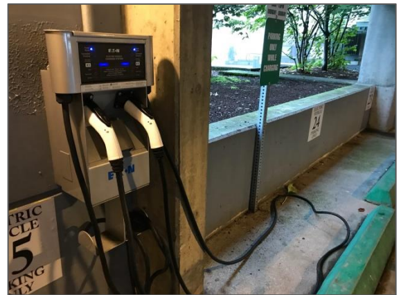
Marine Parking Garage EV Charging Station
