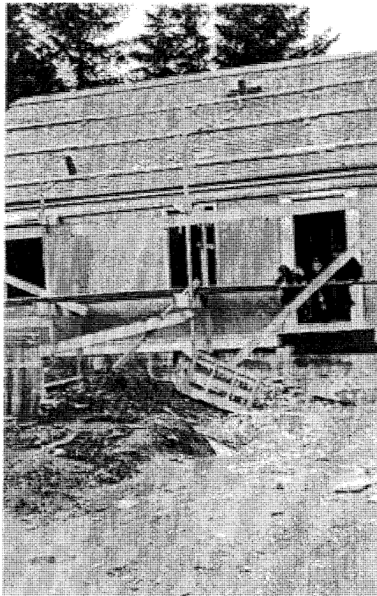
Jimmy Larsen House 10 610 West Eleventh Street Under Construction, ca 1939 Courtesy of Lee Powelson
