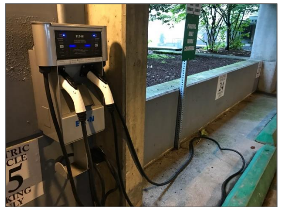
Marine Parking Garage EV Charging Station
