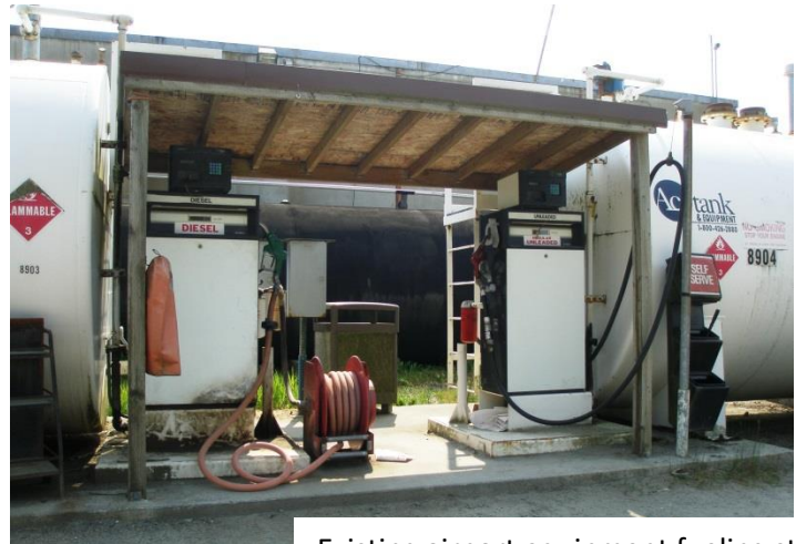
Existing airport equipment fueling station.
