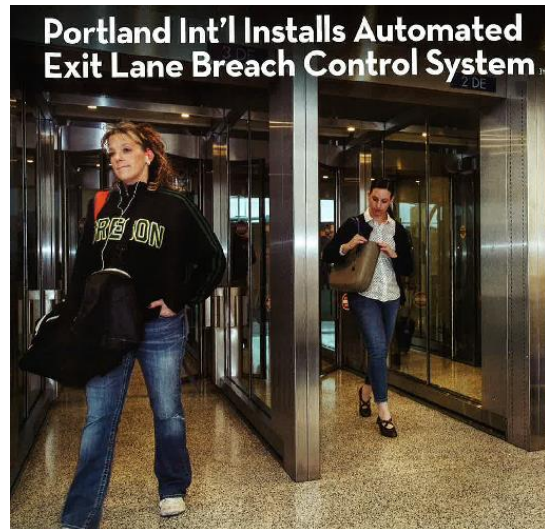
Advertisement image of an automated exit lane system at Portland, OR terminal.
