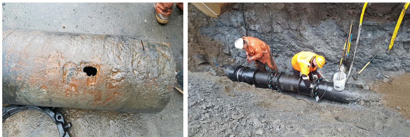
Water main line break and repair near Pt. Lena Loop Road
