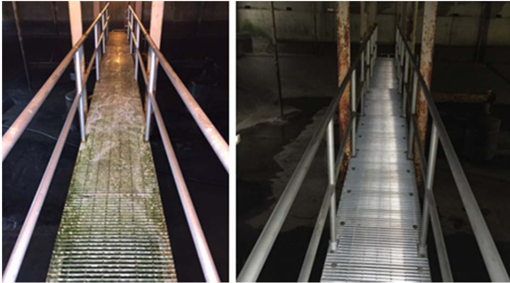
Left to right: JDTP old catwalk over digester; new calwalk and handrails
