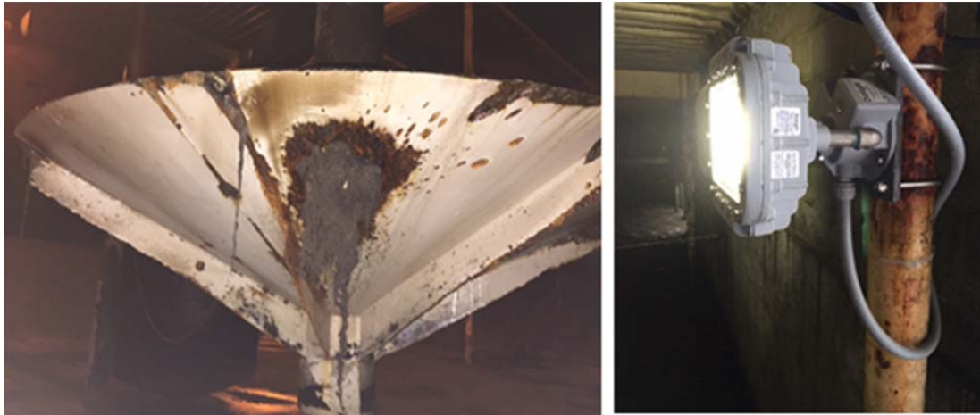
Left to right: JDTP surface impeller condition prior to replacement; new interior LED lighting
