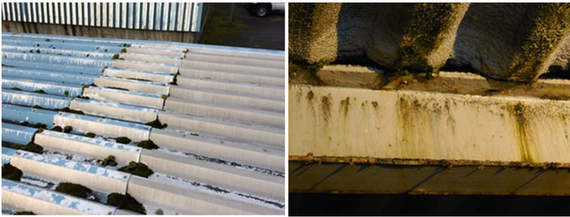
Left to right: exposed exterior fasteners on JDTP digester building roof; interior corrosion to clarifier building roof
