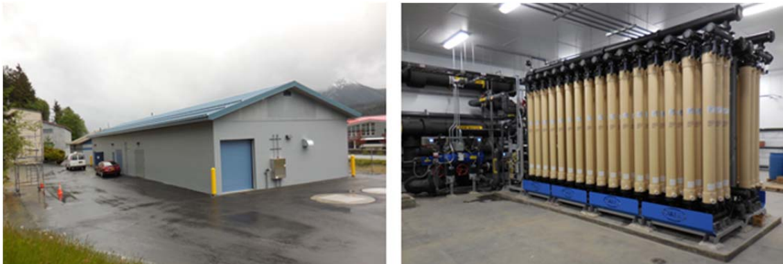
Left to right: new SC water filtration building; new microfiltration membrane units
