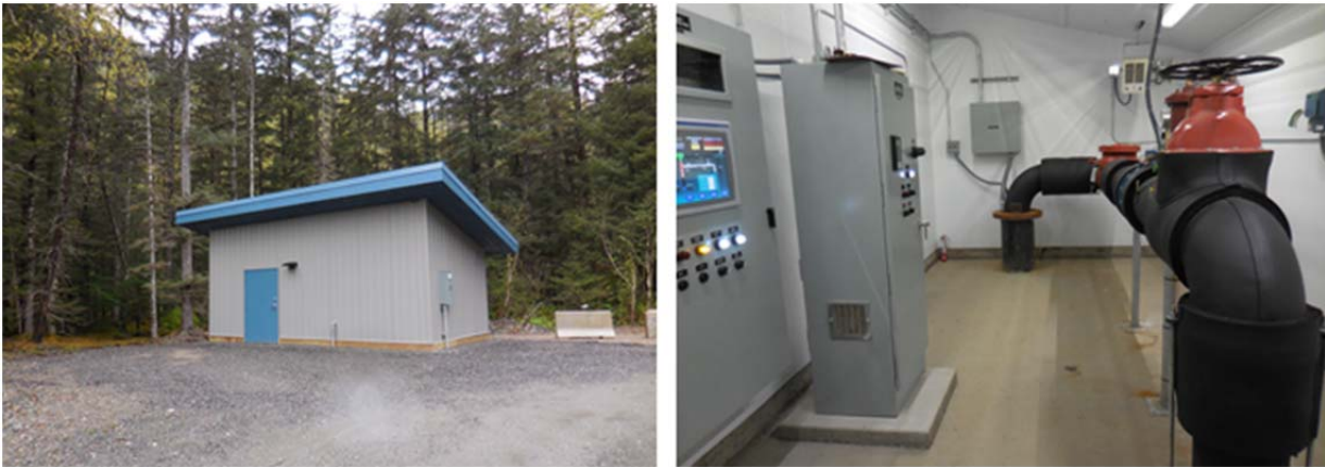
New well house, pumps, piping and controls in well house at LCB
