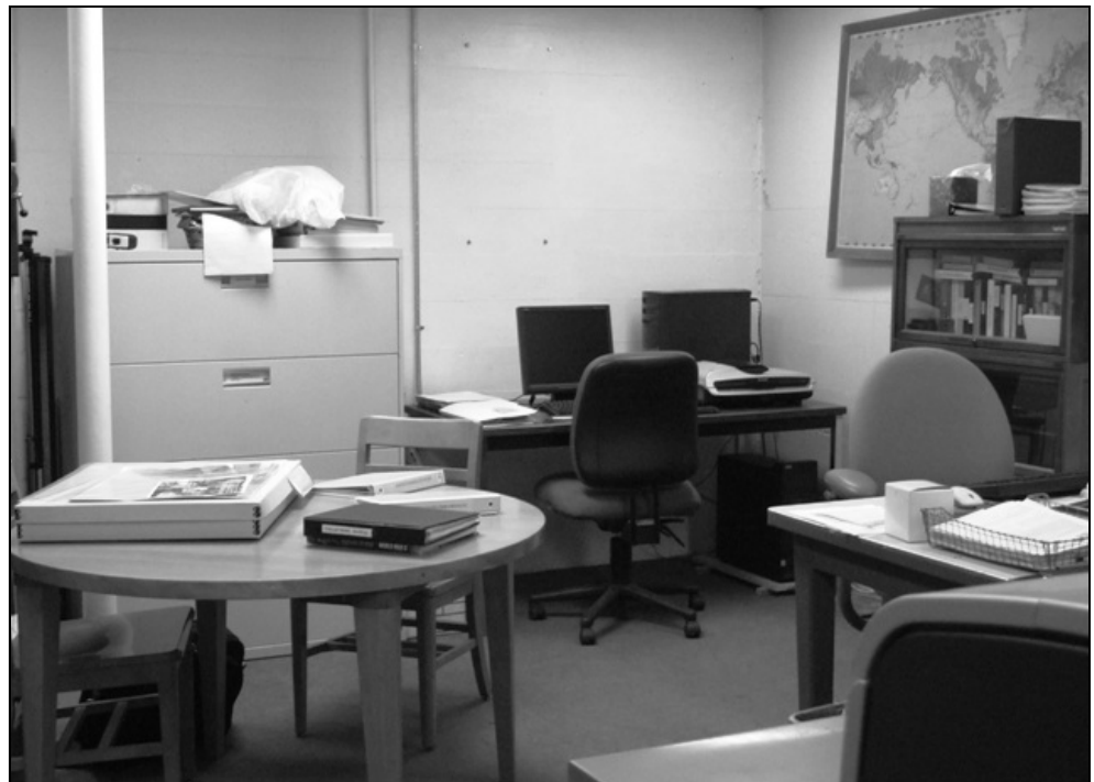
Basement remodel in-progress. Image of reorganized office area and reference library area.
