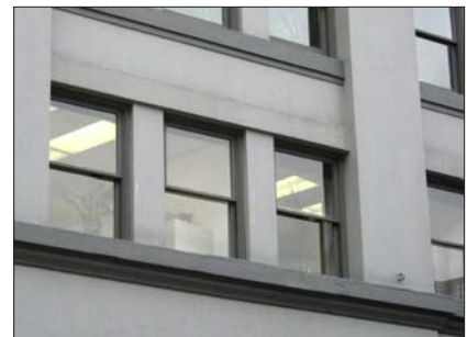
Windows are often grouped in sets of two or three with a pilaster separating them. Note the substantial depth of the detail opening in this building.
