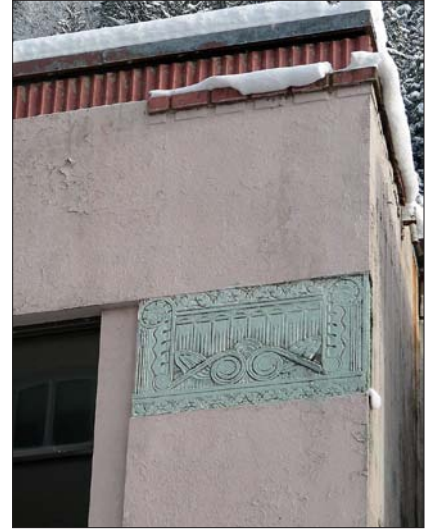
A decorative panel serves as a cap to a vertical attached column, or pilaster, a typical Art Deco detail.
