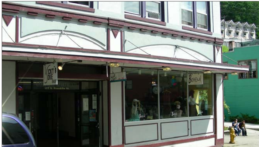
The transoms on the building above have been covered. Although they reflect the openings that were once located there, a more appropriate treatment would be to reopen transoms. Compare with photos on page 15 and 17.
