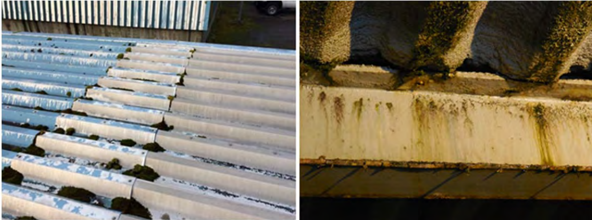
Left to right: exposed exterior fasteners on JDTP digester building roof; interior corrosion to clarifier building roof
