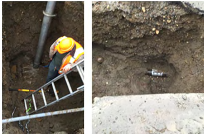
Valley Court mainline leak located and repair sleeve installed
