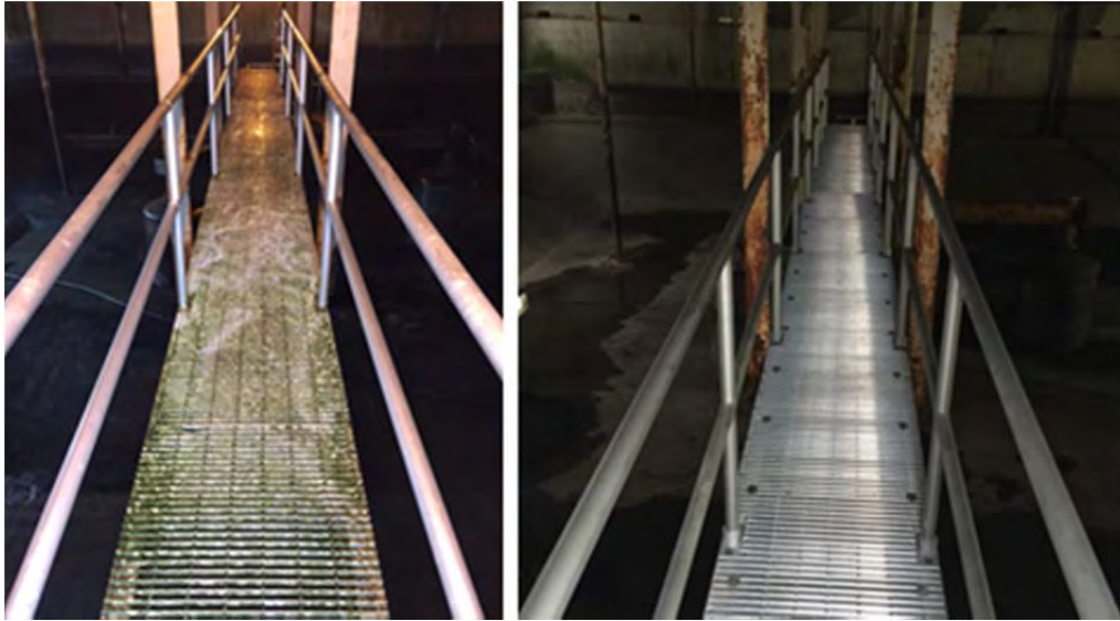
Left to right: JDTP old catwalk over digester; new caltwalk and handrails
