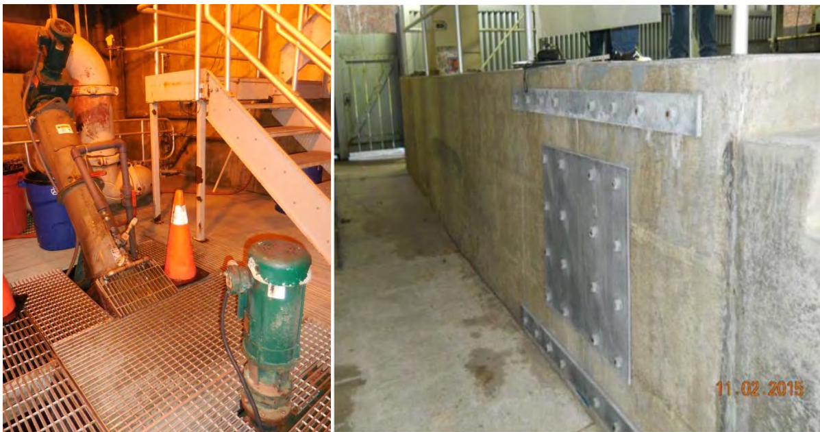
Left to right: MTP existing screening (equipment to be upgraded); JDTP existing influent channel (to be abandoned)
