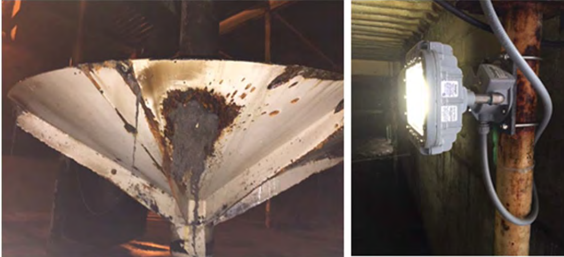
Left to right: JDTP surface impeller condition prior to replacement; new interior LED lighting
