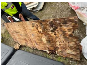
Backside of removed plywood substrate sheet from base of wall.
