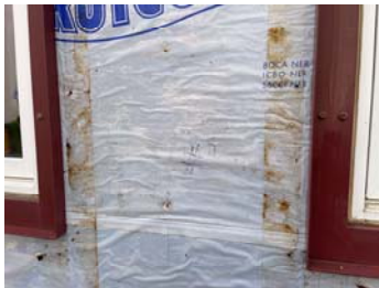
Weather barrier with saturated, plywood substrate beyond.
