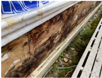
Plywood substrate behind weather barrier with decay and fungus present.
