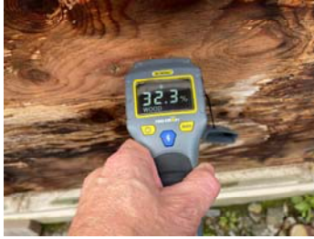
Water damaged plywood substrate with elevated moisture readings.
