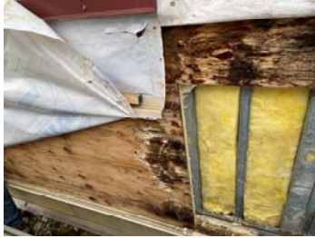
Metal studs and batt insulation beyond polyiso. Batt insulation and studs appeared in good shape.
