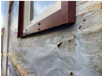
Tears and perforations in weather barrier. Water and fungus visible through weather barrier.
