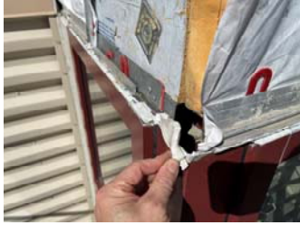
Large hole in the framing, weather barrier and composite metal siding flashing above the storefront corner. Possible cause of water infiltration.
