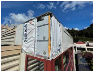
Southwest corner of composite metal panel siding above entry storefront. Weather barrier was discontinuous.
