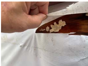
Fungus growth typical all levels of the wall.
