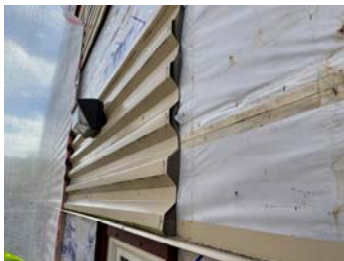
Water stains on the weather barrier surface.
