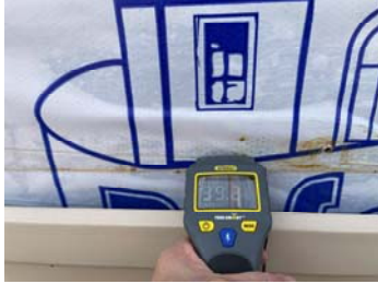
Moisture reading above the exterior light is elevated.
