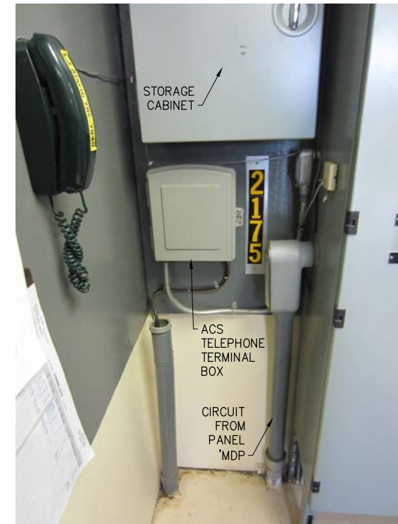
3 (E) ACS SERVICE ENTRANCE E17
