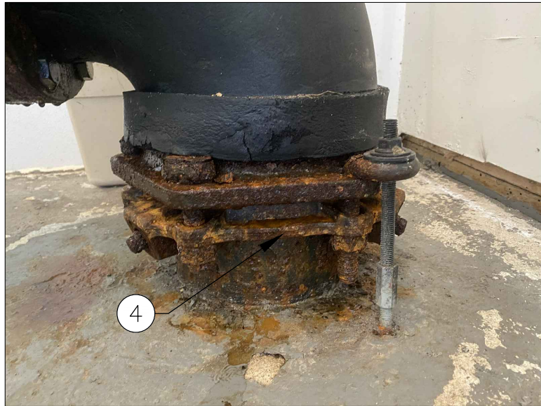
8" DUCTILE IRON SUCTION PIPE
