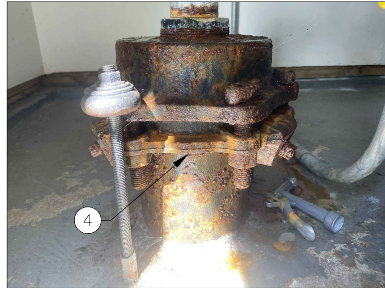
6" DUCTILE IRON DISCHARGE PIPE
