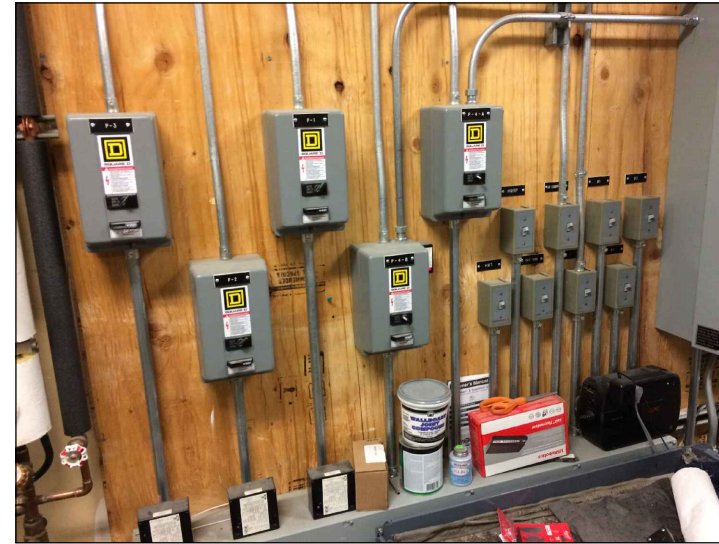
3 M216 Boiler Room 170 Controllers
