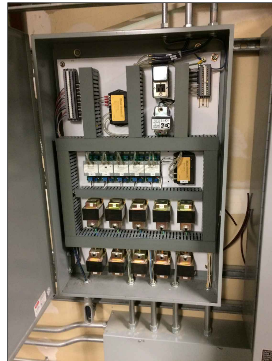
6 M216 Mechanical Room 204 Control Panel IP3
