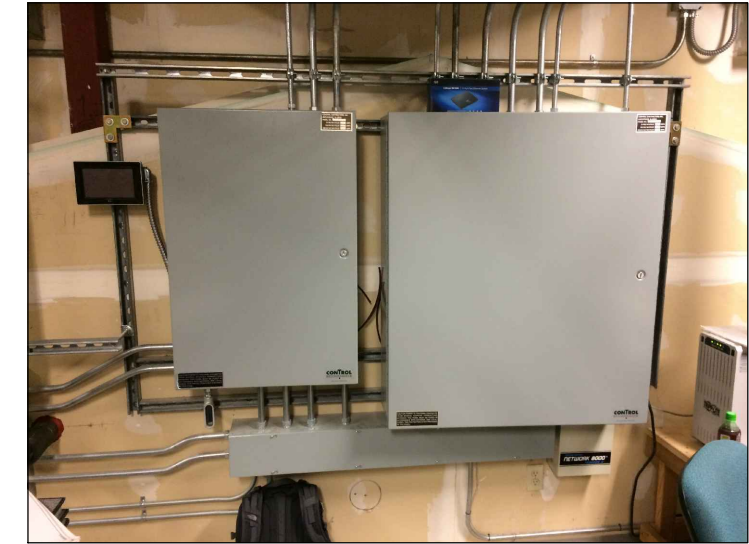
4 M216 Mechanical Room 204 Control Panels
