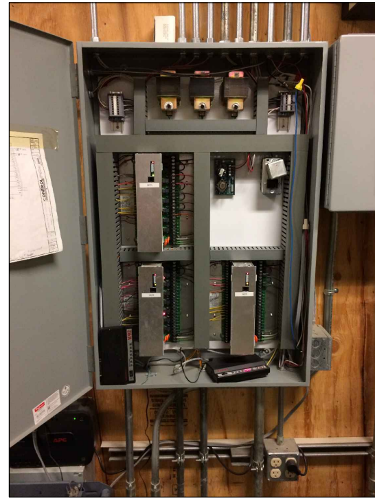
2 M216 Boiler Room 170 Panel IP1
