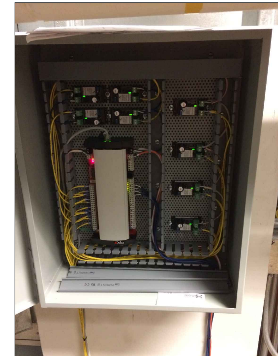
8 M216 Mezzanine Control Panel CP1
