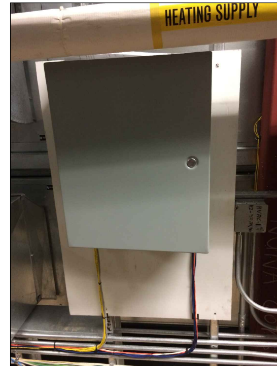
7 M216 Mezzanine Control Panel CP1
