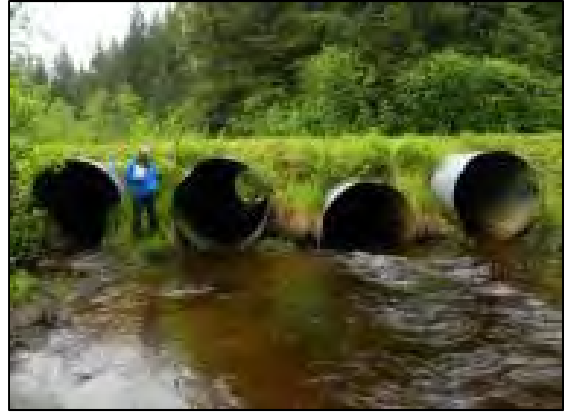
Figure 32. Four side-by-side culverts that create a low and high water velocity fish barrier on a side channel of Montana Creek. Photo courtesy of John Hudson, USFWS.
