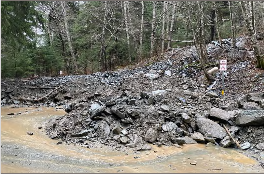
Photo 21: Looking northwest at the Wickersham debris slide, located just past the intersection of Sutherland Drive at the cul-de-sac at the northwest end of Wickersham Avenue (Photo Credit: CBJ Dec 4, 2020; The photo location is shown on Figures 1.4 and 1.5).
