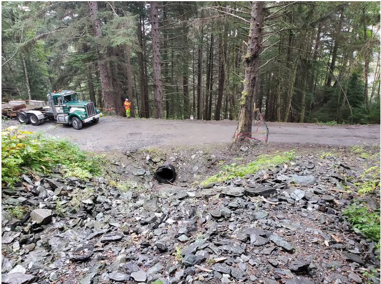
Figure 4: Looking down towards the Gold Creek Flume Trail from the Bathe Creek debris flow gully. Note the large amount of debris in and alongside the gully, as well as the scarring on the tree beside the road that extends to at least 6 feet above ground surface. This gully is very active, and the debris that is deposited at the road crossing is regularly cleaned up. This road crossing has the potential to divert debris flows into the residential community downslope and to the west, especially if more than one surge of debris occurs before the debris can be cleaned.
