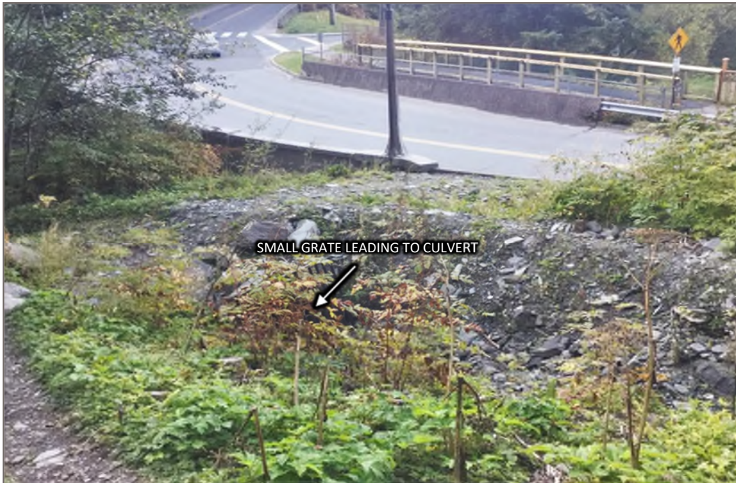
Photo 17: Looking south at debris flow material deposited near the Gold Creek Calhoun bridge. The small grate leading to a drainage culvert indicated and the drainage channel to the grate likely had to be dug out after the event. (Date of Photo: September 10, 2019; The photo location is shown on Figures 1.4 and 1.5).
