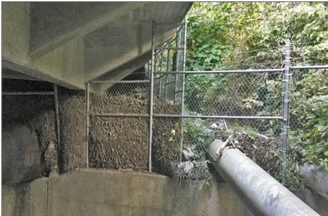
Photo 18: Looking north at debris flow material deposited beneath the Gold Creek Calhoun bridge (Date of Photo: September 10, 2019; The location is shown on Figures 1.4 and 1.5).
