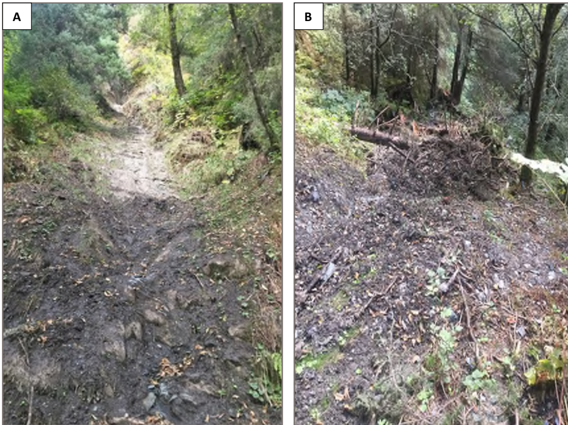
Photo 6: A) Looking northeast and upslope at the gullied path of a debris slide near the northern extent of the study area. B) Looking downslope from the same point as A showing deposited debris (Date of Photos: September 11, 2019; The photo location is shown on Figures 1.4 and 1.5).
