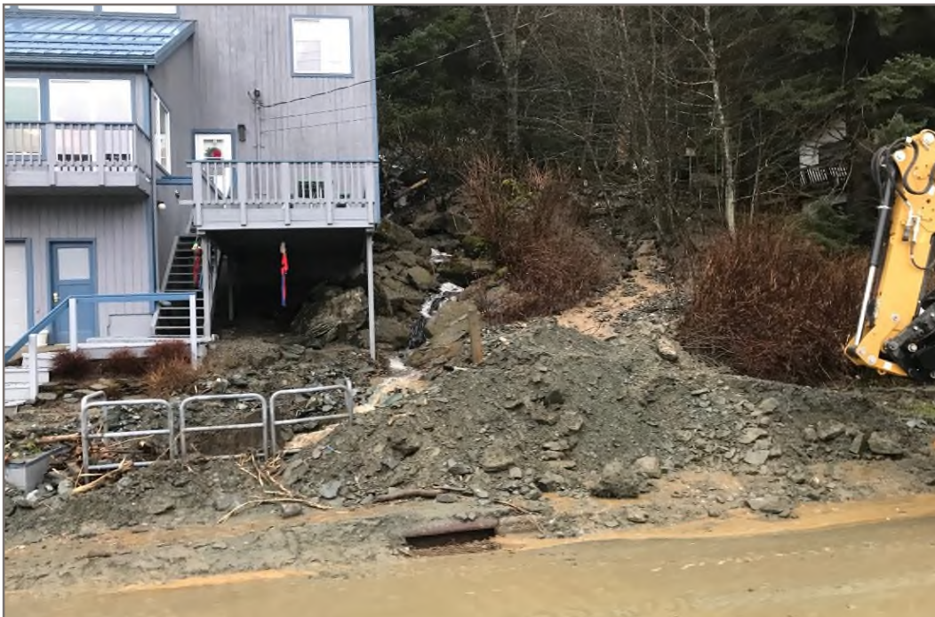
Photo 22: Looking upslope (northeast) at 2020 Glacier Highway at the debris running out onto the road from the Wickersham slide. The guard rail is located at the drainage under the road, which appeared to have been largely plugged by debris (Photo Credit: CBJ Dec 4, 2020; The photo location is shown on Figures 1.4 and 1.5).
