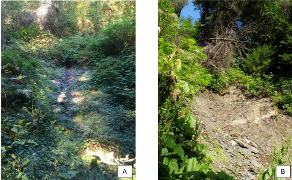
Figure 17: Compare Tetra Tech’s photo from September 10, 2019 (Figure 17A) with residents’ photo from August 1, 2021 (Figure 17B) at the same location. Slope instabilities appear to be ongoing in the historical slide path locations.
