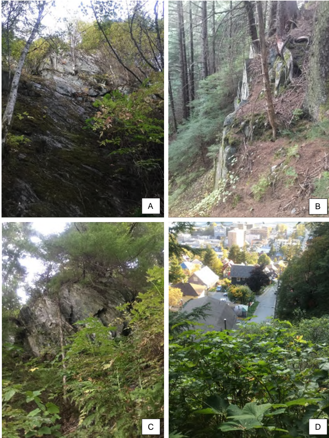
Figure 8: Rockslide track and cliff above rockfall at left-hand blue arrow on Figure 5 (Figure 8A); typical rock bluff above 6 th Street at red arrows on Figure 5 (Figure 8B); rock cliff with detached blocks above corner of 6 th Street and Nelson Street at right-hand blue arrow on Figure 5 (Figure 8C); and talus deposit below rock cliff, 6 th Street visible below (Figure 8D).
