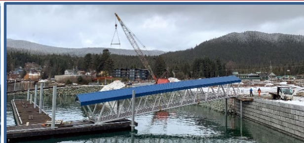
This picture shows the newly installed gangway by Trucano Construction at the Statter Harbor For Hire Facility Phase III (b). The project completion date is scheduled for May 2021. Photo by Matthew Sill
