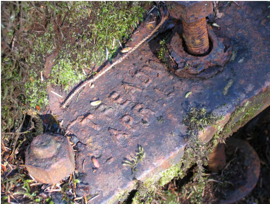
Part of Metal Lathe with foundry mark indicating it was cast at the Treadwell Foundry. Photo taken in April 2010, courtesy of Wayne Jensen
