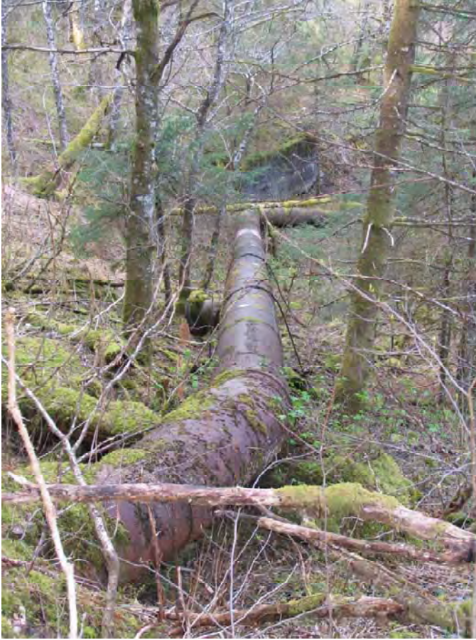
Pipeline to 240 Mill from Treadwell Ditch Photo by Wayne Jensen
