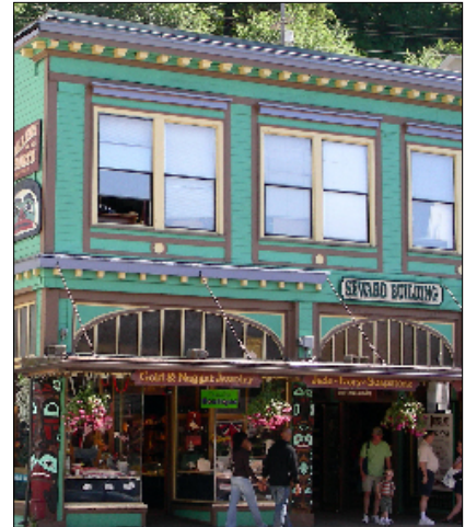
The Seward Building (1913, 145 S. Franklin Street) has a decorative cornice, recessed entry and facade detailing characteristic of a Late Victorian Style.
