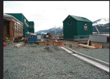
The parking lot on the north side of Taku Fisheries building was reconstructed with a new layout.
