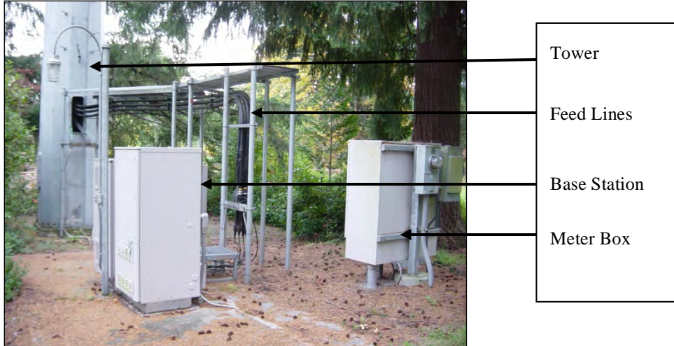
Figure 1: Example of 1900 MHz Wireless Infrastructure Ground Equipment
