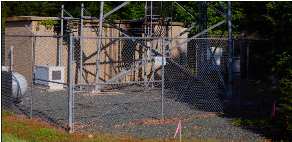
Figure 2: Example of 800 MHz Base Station
