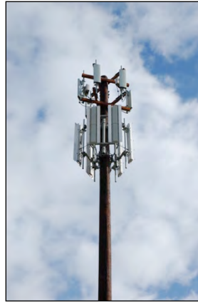
Sectorized (panel) Antenna Array
