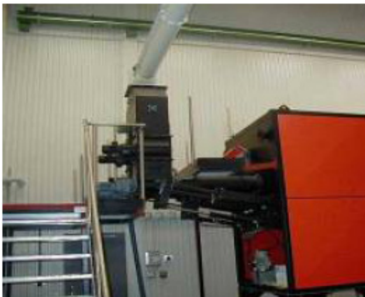
FIGURE 4 BioCon-ERS Incinerator Furnace
