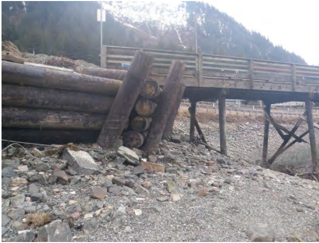
Figure 5: Failed timber retaining wall under north approach dock
